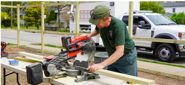
The HHK Community Garden under construction by the Ho-Ho-Kus DPW. Photo by: Councilman Dane Policastro.
