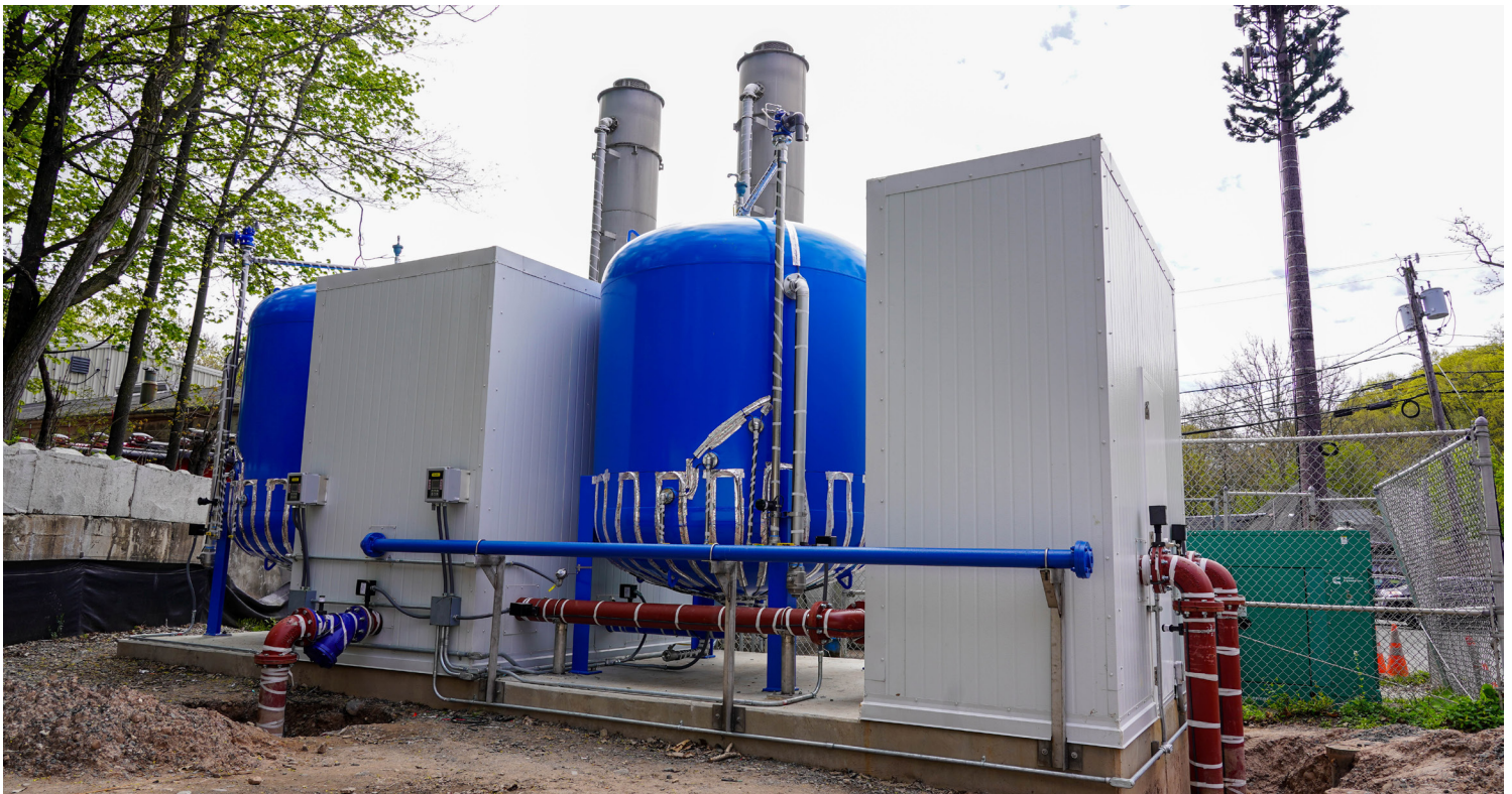
One of the four PFAS treatment facilities in Ho-Ho-Kus. HHK water is now below detectable levels for both PFOA and PFNA contaminants throughout our water system. For additional information please visit the Borough website hhkborough.com . Photo by: Councilman Dane Policastro.
